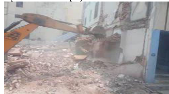
Fig 2 : Demolished site of Meraj Colony
