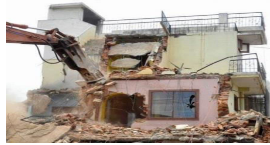
Fig 1 : Demolished site of Murad Nagar
