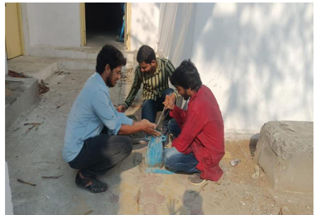
Fig 7: Tampering of concrete
