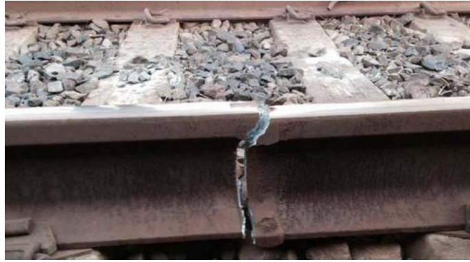
Figure 1. Crack in Railway Track.
