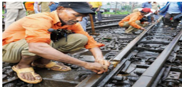
Figure 2: Traditional Railway Track Crack Detection.
