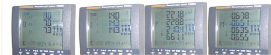
Figure 2. Values recorded by the local equipment (U, I, P, λ)
