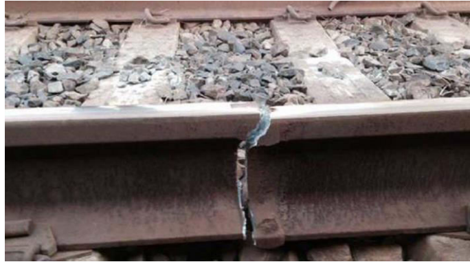
Figure 1. Crack in Railway Track.
