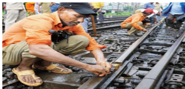
Figure 2: Traditional Railway Track Crack Detection.
