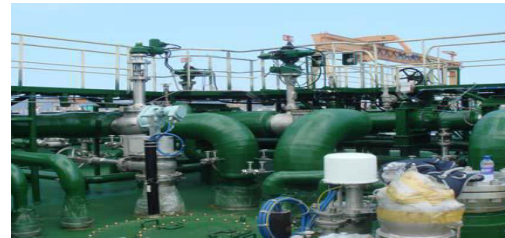
Figure 1 Photo of the valves are installed on vessels
